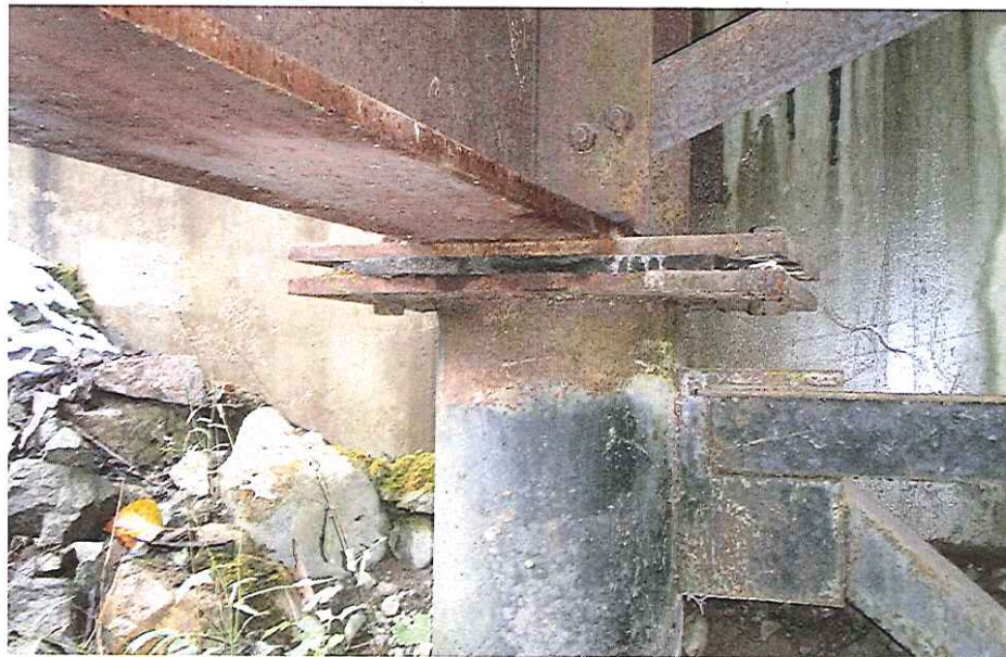
CK-2042 Condition of Bearing pads (buldging out)
